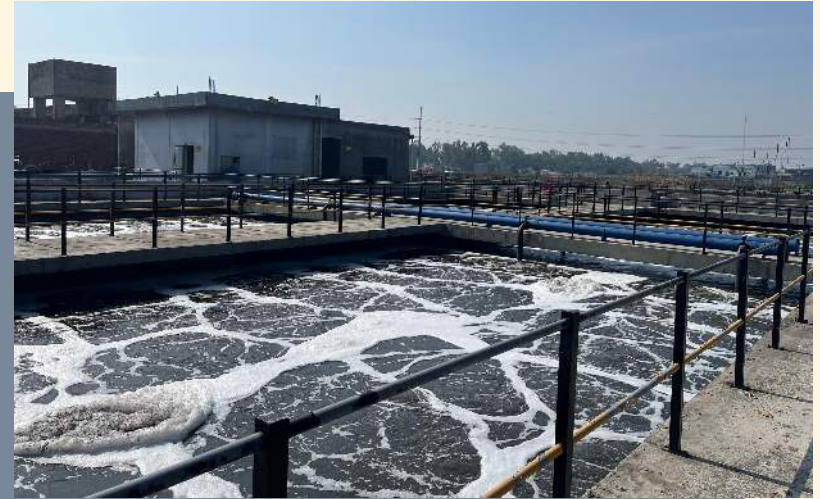
Illustration: Wastewater treatment at a supplier of BRANDS Fashion
